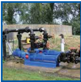
Transfer pumps at a WWTW's pumping sludge
