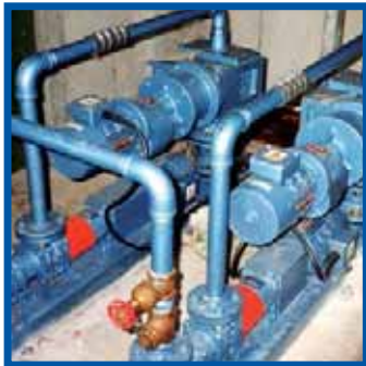
Packaged pumping system transferring raw sewage
