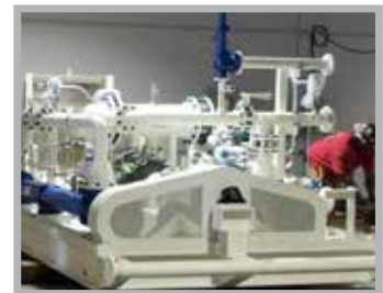
Closed Drain - Knock Out Drum liquor hydrocyclone feed pumps
