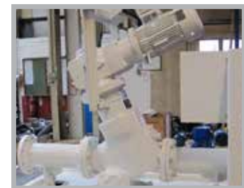
Sewage maceration and discharge from an offshore platform
