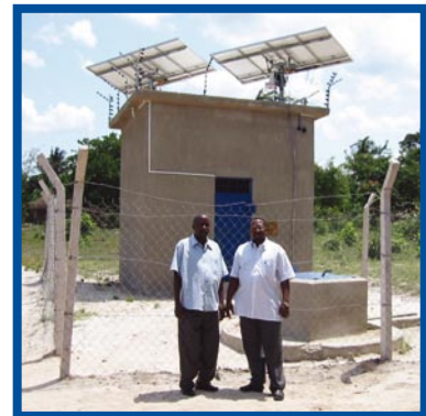
The solar arrays installed on the pump house with security fencing to prevent theft.
