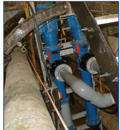
Vertical pumps installed in a 47m deep tunnel
