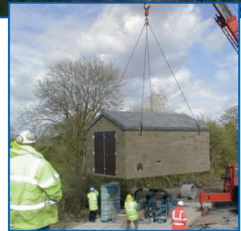
The management of craneage for a contract to install a special acoustic GRP kiosk and sewage pumps
