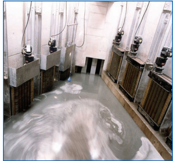
Installation of nine Discreens and two Munchers, together with a guide rail system for easy removal from the 7 metre deep storm chamber
