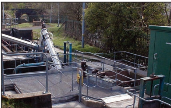
Extractor, screen and macerator installation
