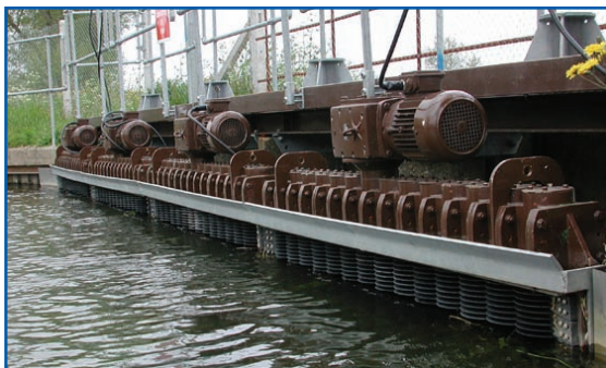
4 Discreens supplied and installed on a lagoon intake
