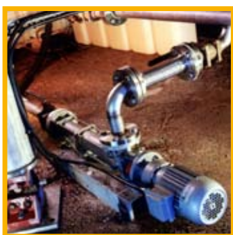
Transfer pump for water softening agents and sodium hydroxide liquor
