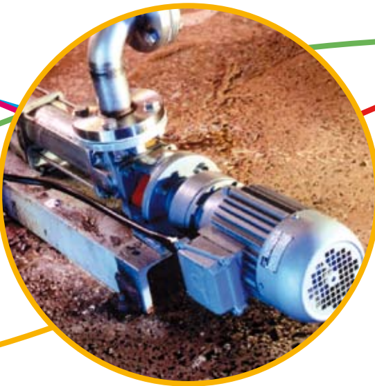
Transfer of industrial detergents
