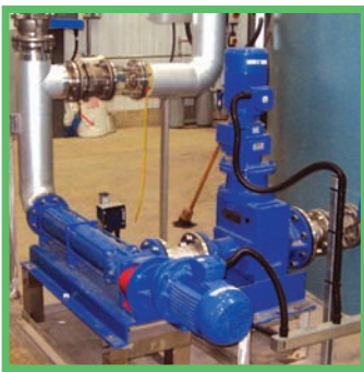
Transfer pump and Muncher for biodegradable waste
