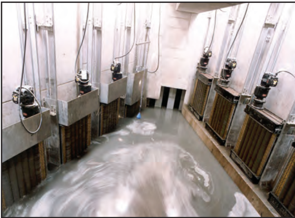
Nine Discreens installed in a stormwater pumping station
